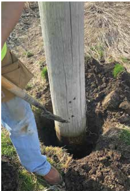
Regular testing of poles is a critical component of system maintenance. Any deemed to be defective are replaced.
