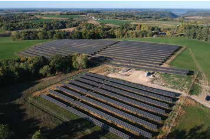
The Bluff Prairie Solar array located by Red Mound in Vernon County.
